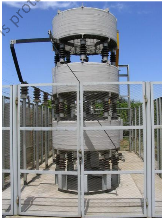
Figure 2.6 : A 3-phase core-less or air-core Shunt Reactor (Rocha and Mendes, 2006)
