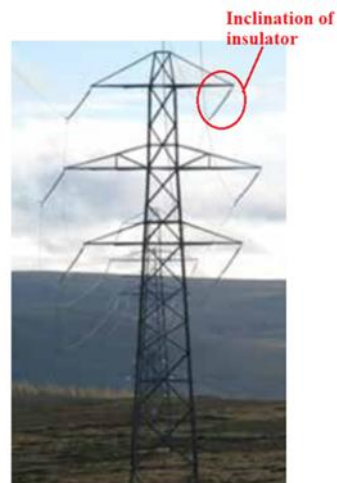
Figure 1: Inclination of insulation due to wind load
