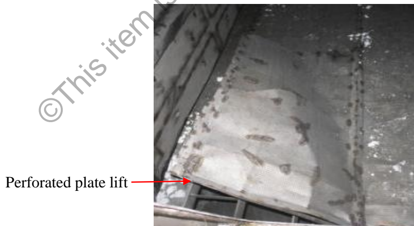
Figure 1.3: Perforated plate lift off due to joint failure.
